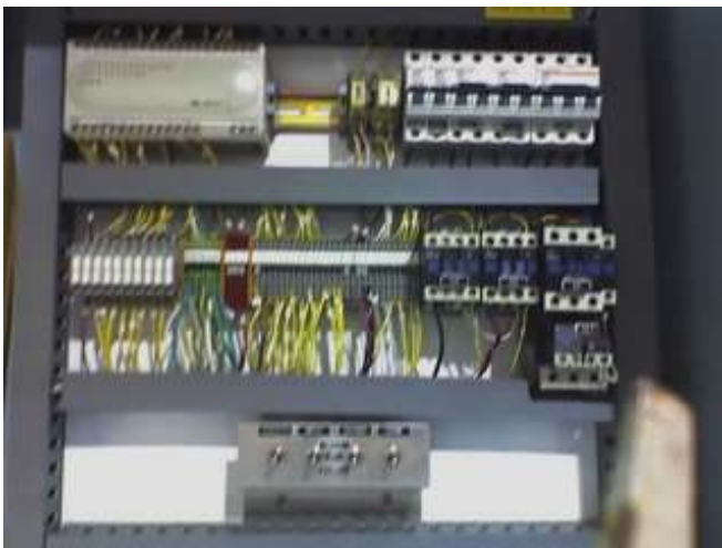
Figure 5: PLC and Monitoring System
